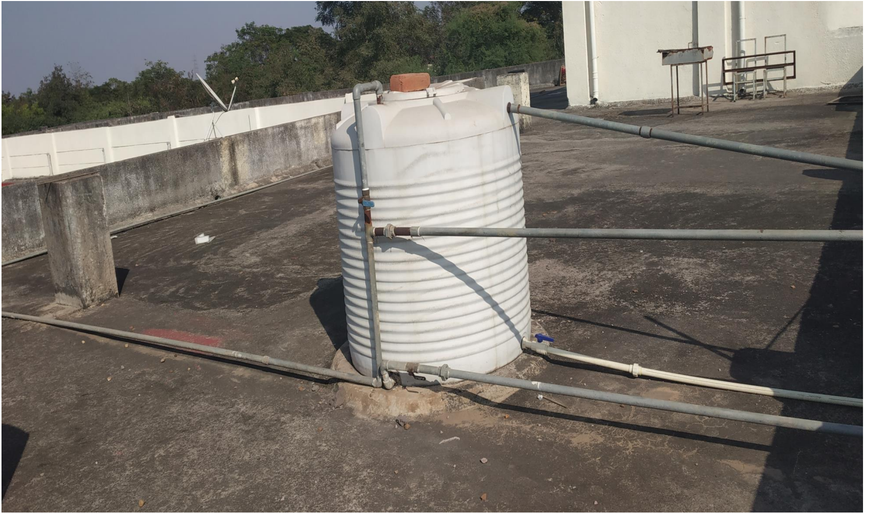
WELL MAINTAINED OVERHEAD TANK WATER DISTRIBUTION SYSTEM
