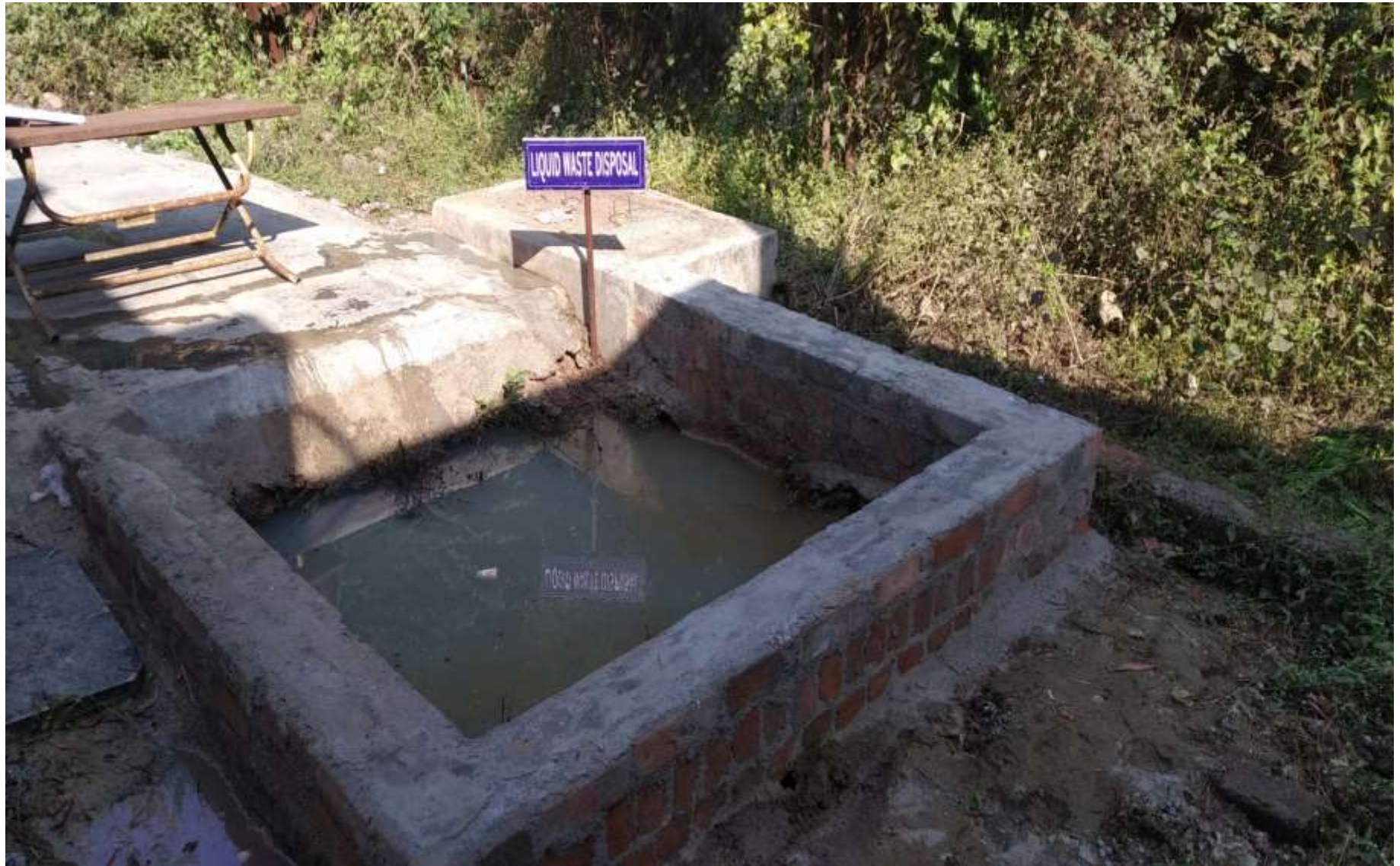
LIQUID WASTE PIT
